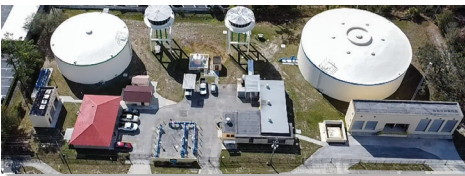
The Water Treatment Plant pictured is located at 9748 Decubellis Road.
